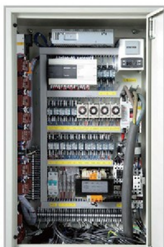
■ Electrical Cabinet with Mitsubishi PLC
